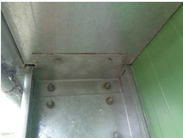
Rust developing on folded steel cleat
