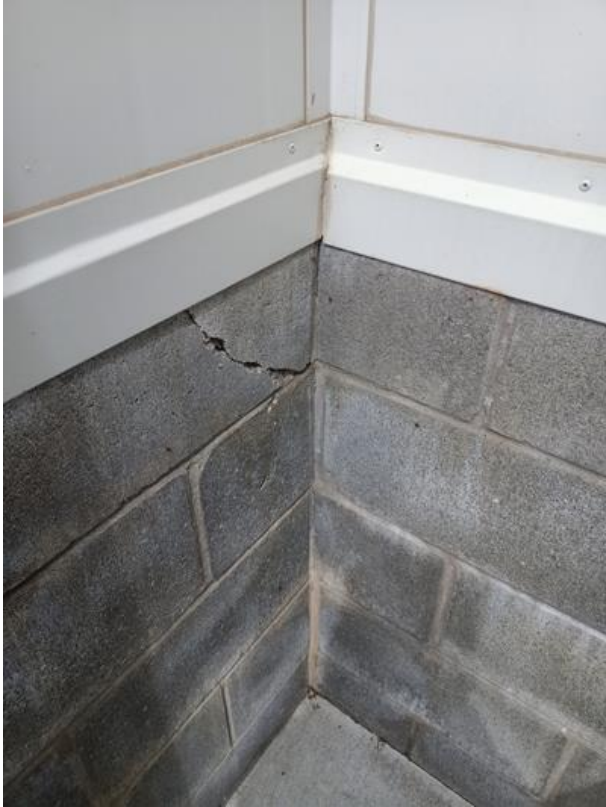
Cracked concrete block.
