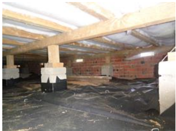
Subfloor - insulation and pvc sheet.
