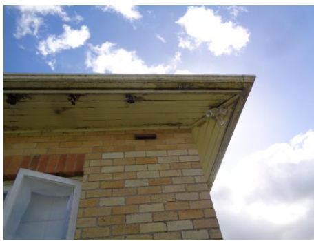
Grime to soffit and gutter
