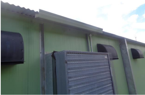
Intake ducts and extract louvres
