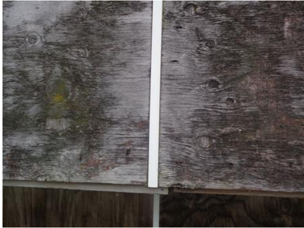
Plywood in poor condition
