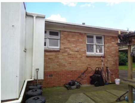
Timber joinery poor condition
