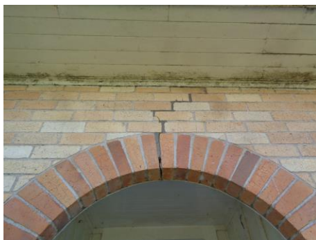
Crack to brick work at entry arch.
