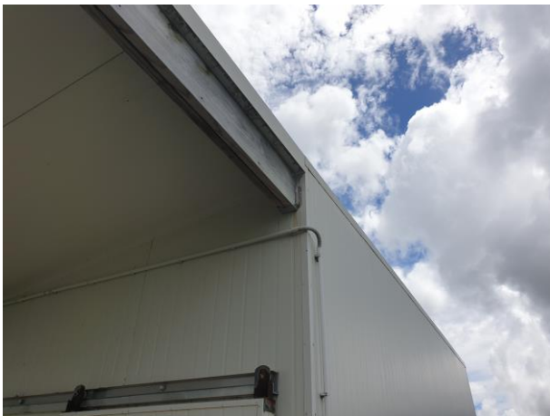
Light weathering to exposed timber beam
