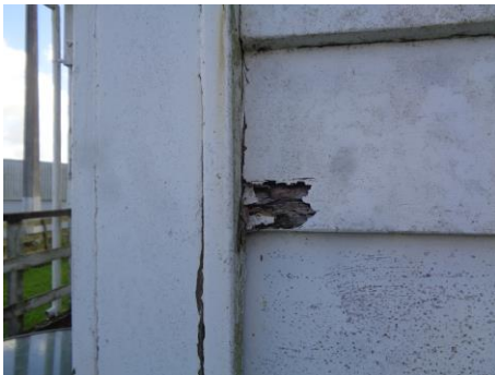
Rot to weatherboard
