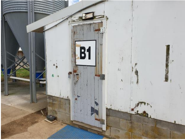
Typical weathering of exterior cladding and doors
