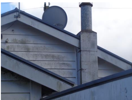
Cracks to chimney
