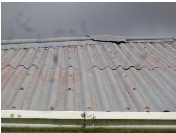
Roofing nails old lead head type – replace.
