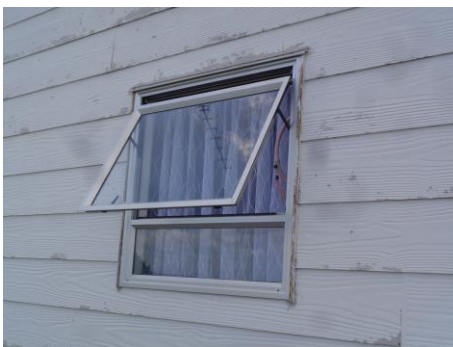
Timber scribe in poor condition
