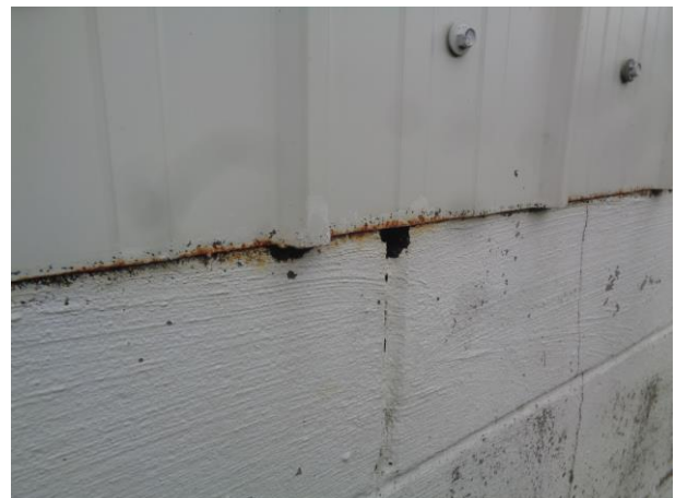
Rusting of cladding at lap with concrete
