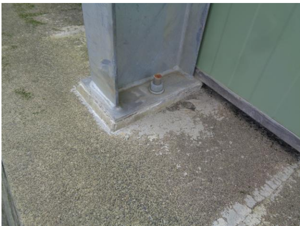
Insulated panel close to concrete slab and not located on a concrete nib.
