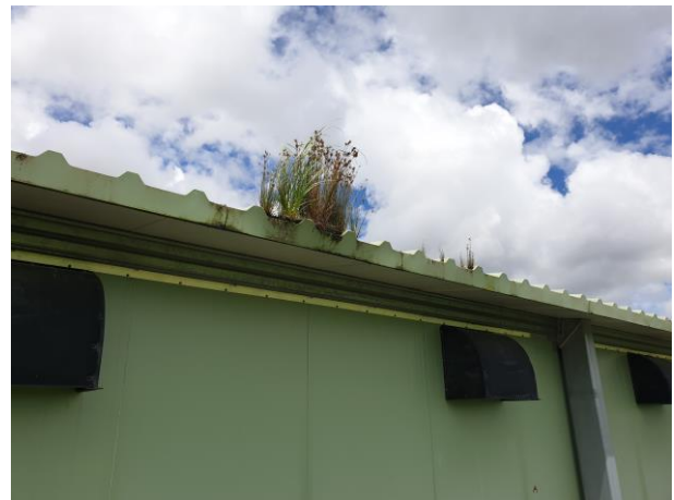
Vegetation growing in the gap between the roofing and the end cap flashing
