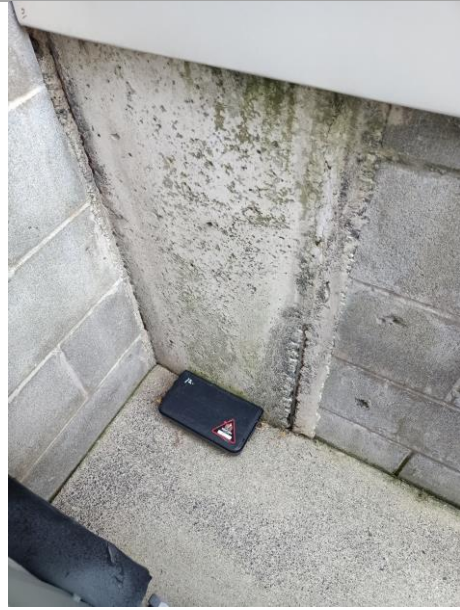
Reinforcing bar visible at insitu concrete
