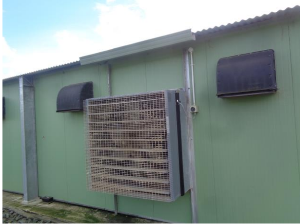
Intake ducts and extract louvres.
