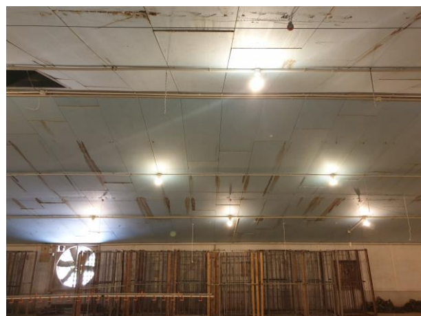
Typical interior construction Typical ceiling lining damage
