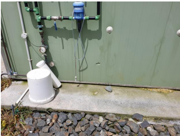
Minor wall damage
