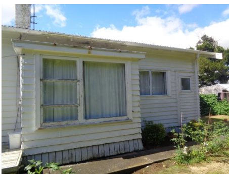
Timber window poor condition
