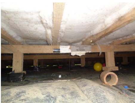
Subfloor – insulation and pvc sheet.
