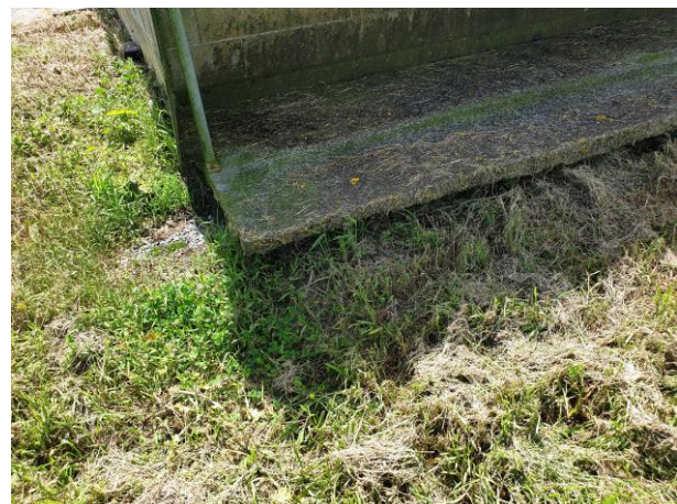
Typical partial undermining of exterior slab
