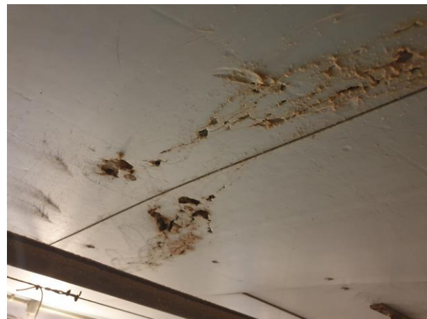
Typical ceiling lining damage
