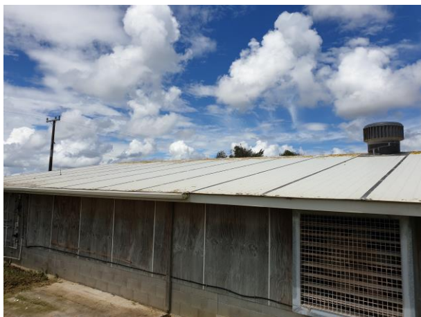
Lichen growth on roofing
