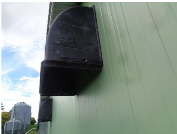
Intake ducts and extract louvres. Louvres to black intakes missing or damaged.
