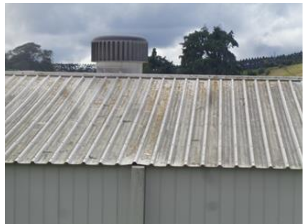
Roof has lichen and grime.
