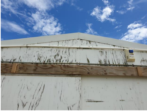
Typical weathering of exterior
