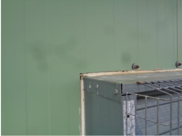
Poor installation detail around louvre frame
