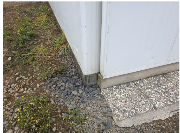
Minor slab/foundation crack
