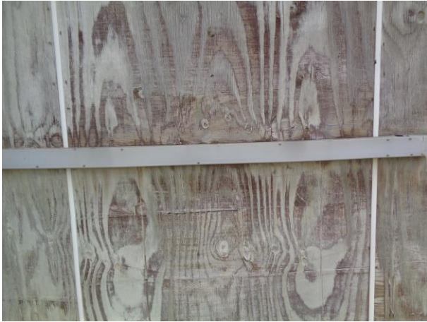
Plywood in poor condition
