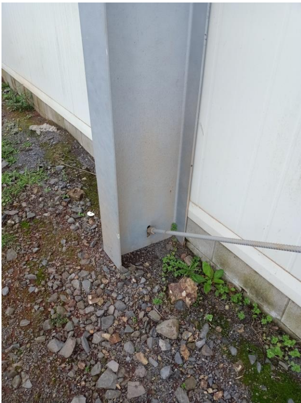
Column base plate to be exposed, condition inspected and remedial work undertaken if required. Base plate to remain exposed and not buried in ground.
