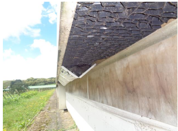
Poor repair to vent grille.
