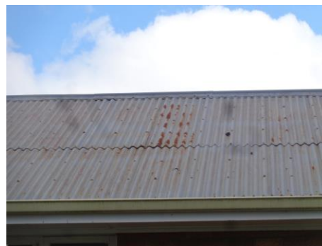
Roofing iron surface rust
