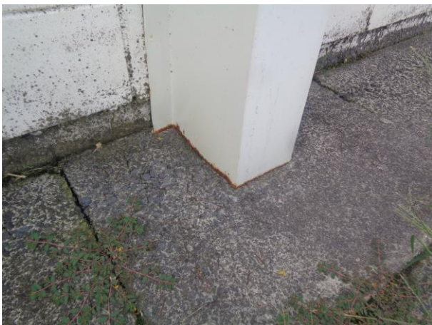
Rusting of column cover flashing.
