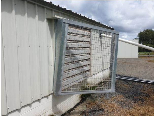
Dislodged ventilation screen
