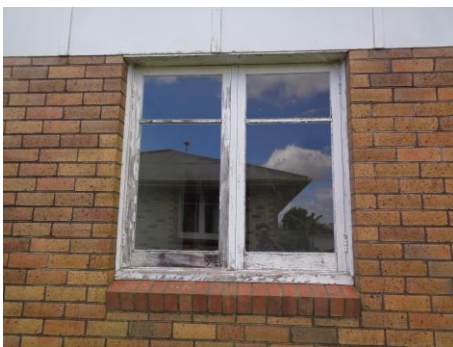
Timber joinery in poor condition.
