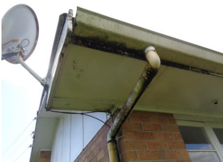
Grime to soffit, gutter and downpipe
