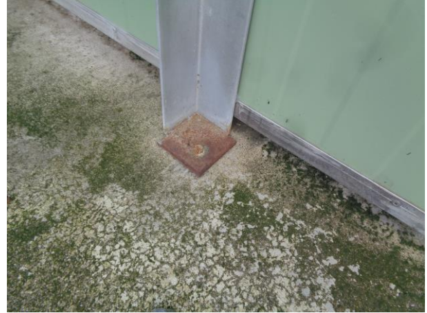
Rust to extract louvre frame
