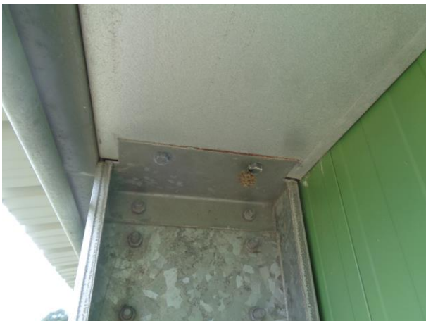
Rust developing on folded steel cleat
