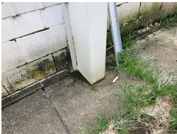
Corrosion of Colorsteel flashing around external columns
