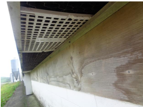
Poor repair to vent grille and plywood with no protective coating.
