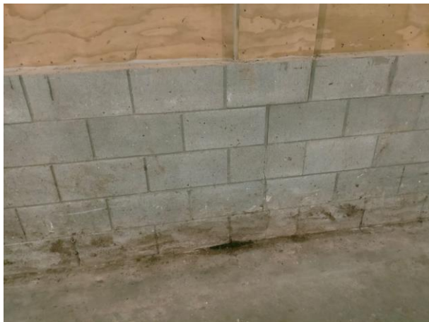
Typical vertical shrinkage cracking in perimeter block walls
