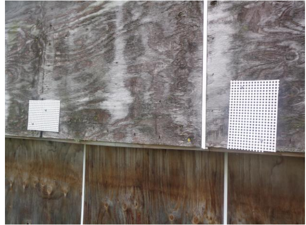
Poor repairs to holes in plywood.
