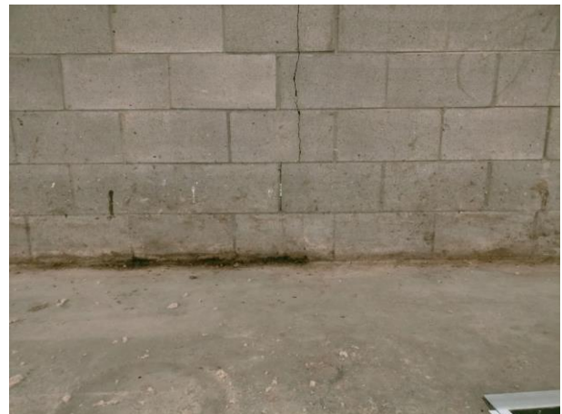
Full thickness vertical shrinkage crack in perimeter block wall
