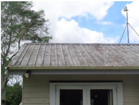
Odd appearance of roof – investigate condition
