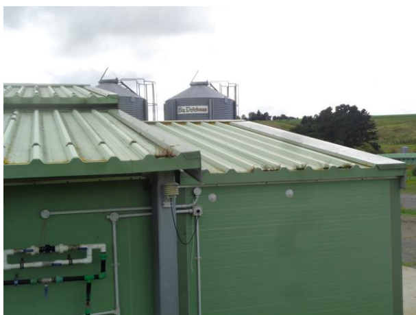
Vegetation growing at insulated panel end caps
