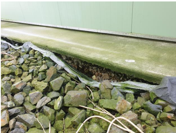
Typical undermining of perimeter slab
