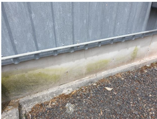
Typical perimeter upstand wall cracking and mould
