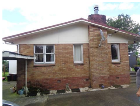
Barge board in fair condition
