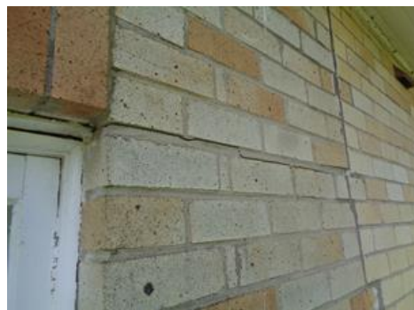
Crack to brick work of extension
