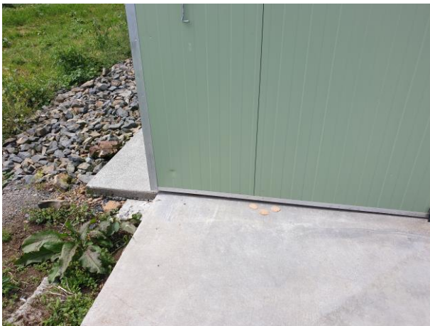
Minor wall damage
