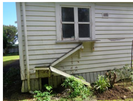
Timber window poor condition.
