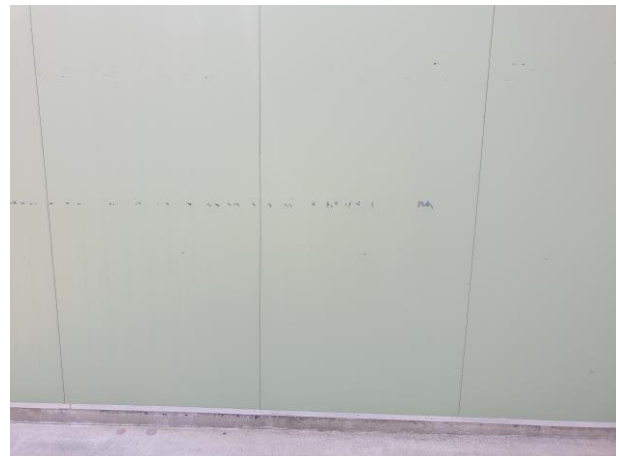
Localised areas of minor wall damage
