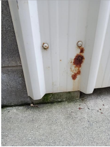
Corroded metal cladding at lap over concrete.
