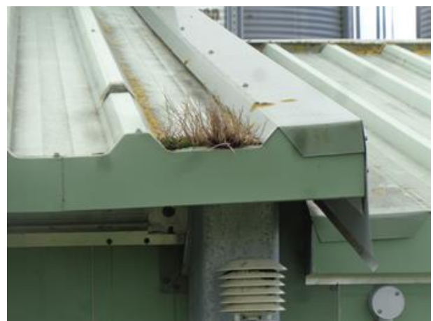
Vegetation growing at insulated panel end caps
