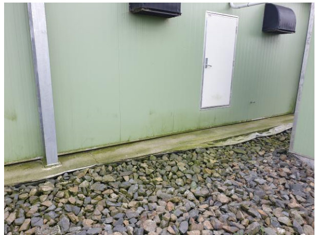
Minor perimeter slab cracking and green mould
