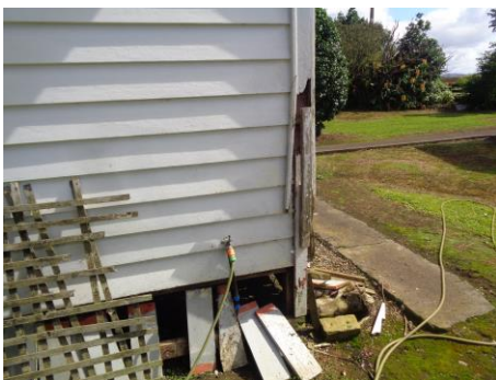
Rotten timber corner facing
