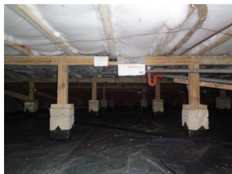
Subfloor insulation and pvc sheet.
