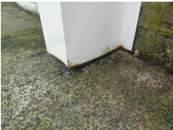
Rusting of column cover flashing.
