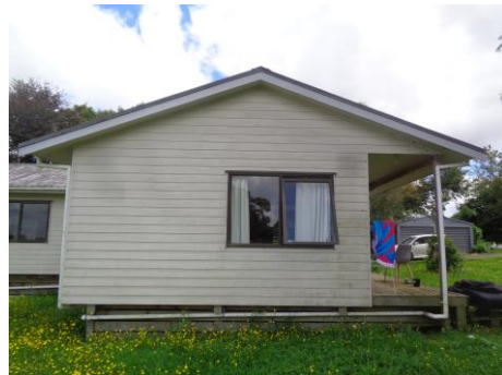
Grime to walls
