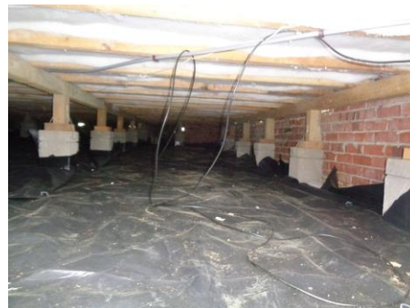
Subfloor – insulation and pvc sheet.
