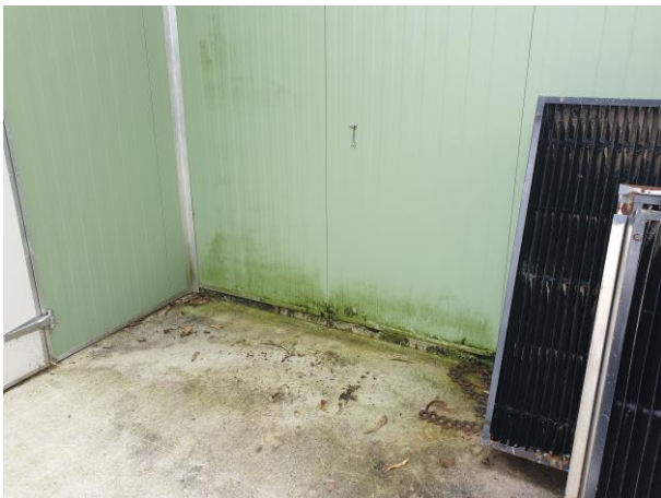
Localised areas of mould
