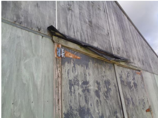
Ineffective door head flashing
