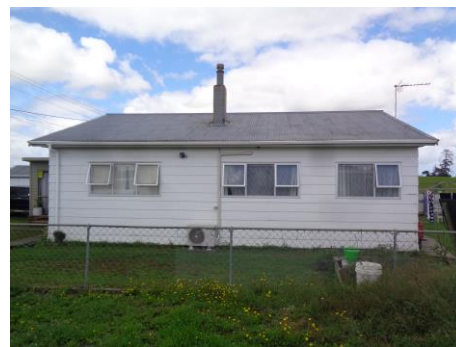
Roof showing signs of wear.
