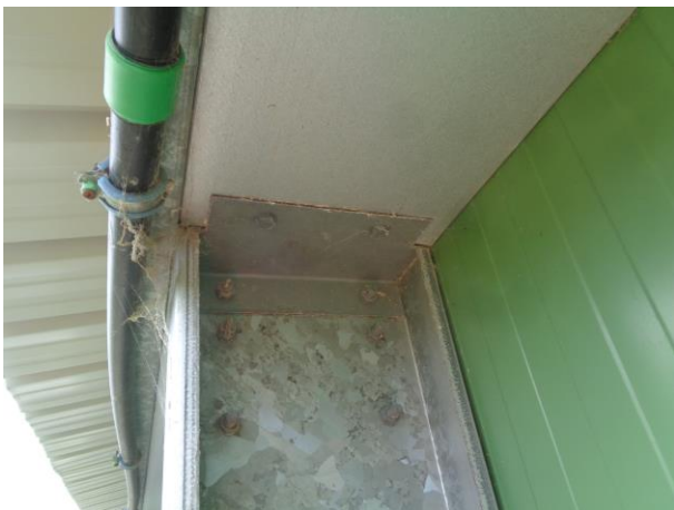
Rust developing on folded steel cleat
