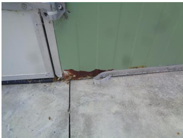
Rust to insulated panel at interface with concrete paving.
