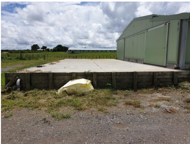
Timber pole retaining wall to rear yard slab showing minor damage to posts and rails
