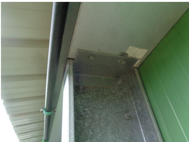
Rust developing on folded steel cleat
